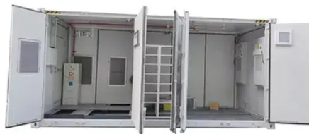
1075KW HH ESS
